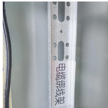
Battery Energy Storage Systems (BESS) . BMarko
