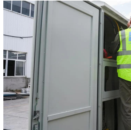
Energy storage container, BESS container
