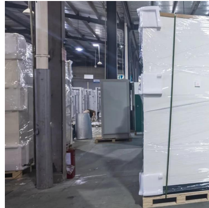
Energy storage container, BESS container
