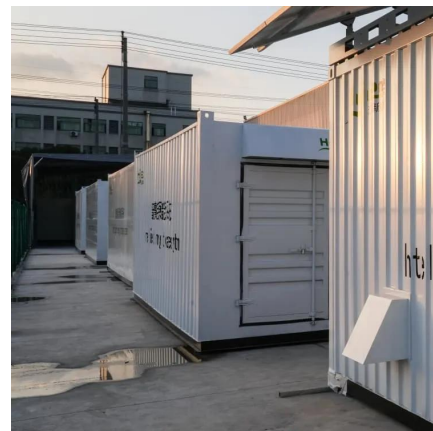
Energy storage container, BESS container
