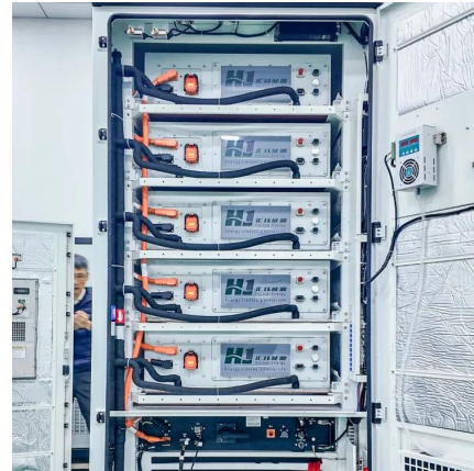
Energy storage container, BESS container
