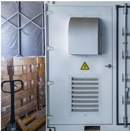
Battery Energy Storage System Container ...
