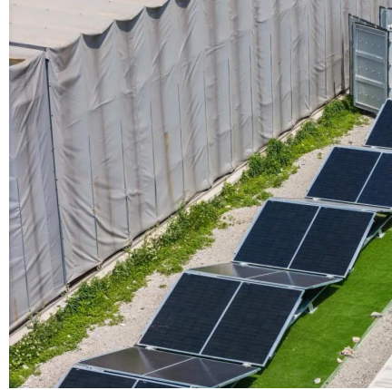
Photovoltaic micro inverter company in Gothenburg Sweden
