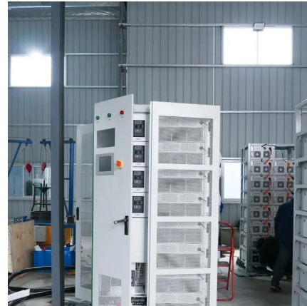
Energy storage container, BESS container
