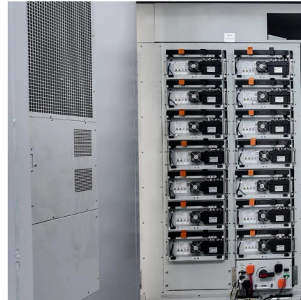
Energy storage container, BESS container
