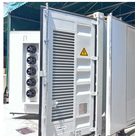
Energy storage container, BESS container
