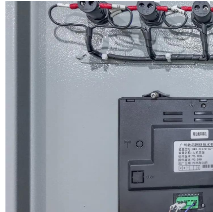
GRL DNHLX-PV12 / 1 DC solar combiner box
