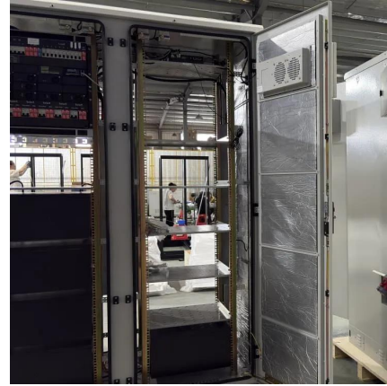
Energy storage container, BESS container
