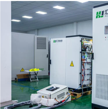
Energy storage container, BESS container
