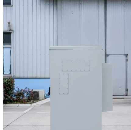
50 kw 50kw Off Grid Solar Hybrid System on Grid 20kwt ...
